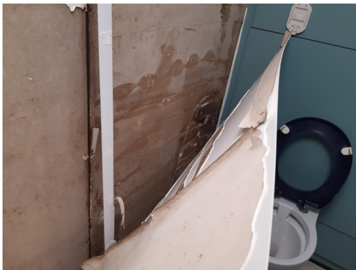
Leak in patient toilet in CF unit
